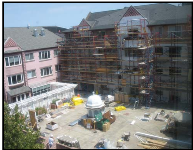
Construction is currently taking place on the west side of the Waterford building.
